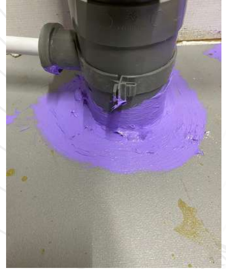
5.1.4 Soil stack through floor
