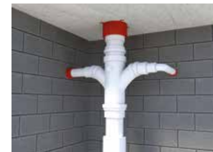
Pipework and Trunking
