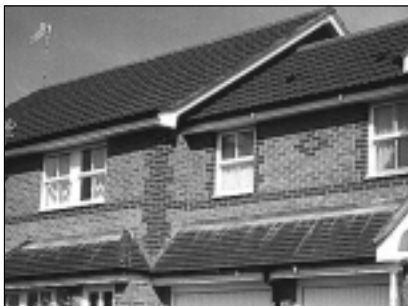
Roof tiles spoiled by run-off staining.
