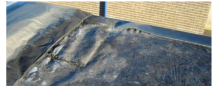
Defects require remedying
