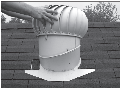
1. Remove old turbine from its base. 2. Place new turbine head over existing base with brackets on the outside of the base.
